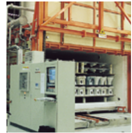
Pressure regulator on excess air burners in the ceramics industry
